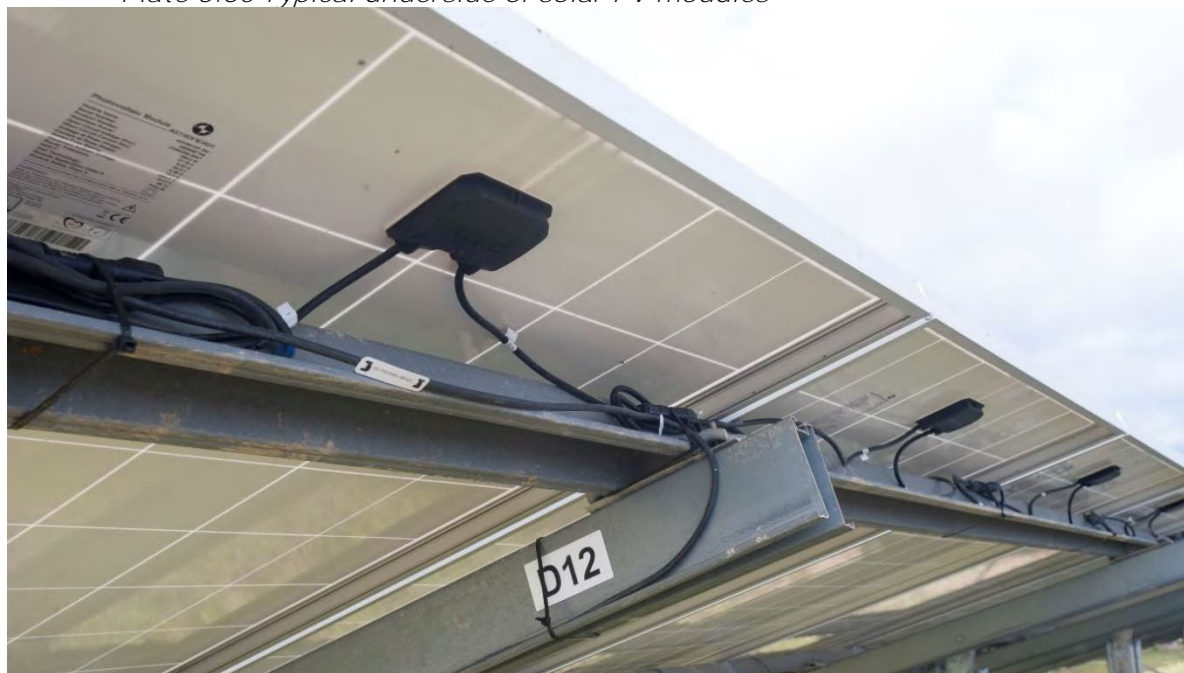
Plate 5.5c Typical underside of solar PV modules
