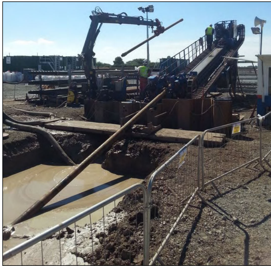
Figure 3.23: HDD rig carrying out landfall works at the Westermost Rough offshore wind farm.
