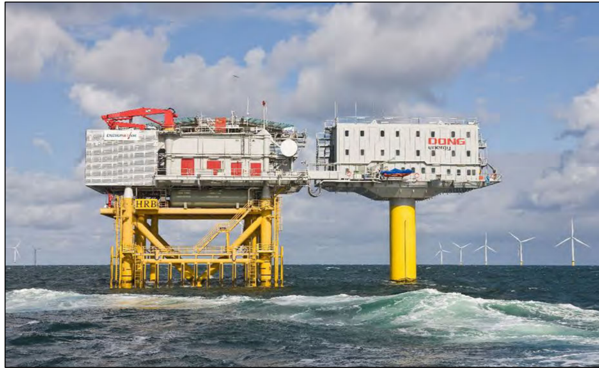
Figure 3.16: Offshore accommodation platform (right) at the Horns Rev 2 offshore wind farm, sited next to an offshore substation (left) 2 .
