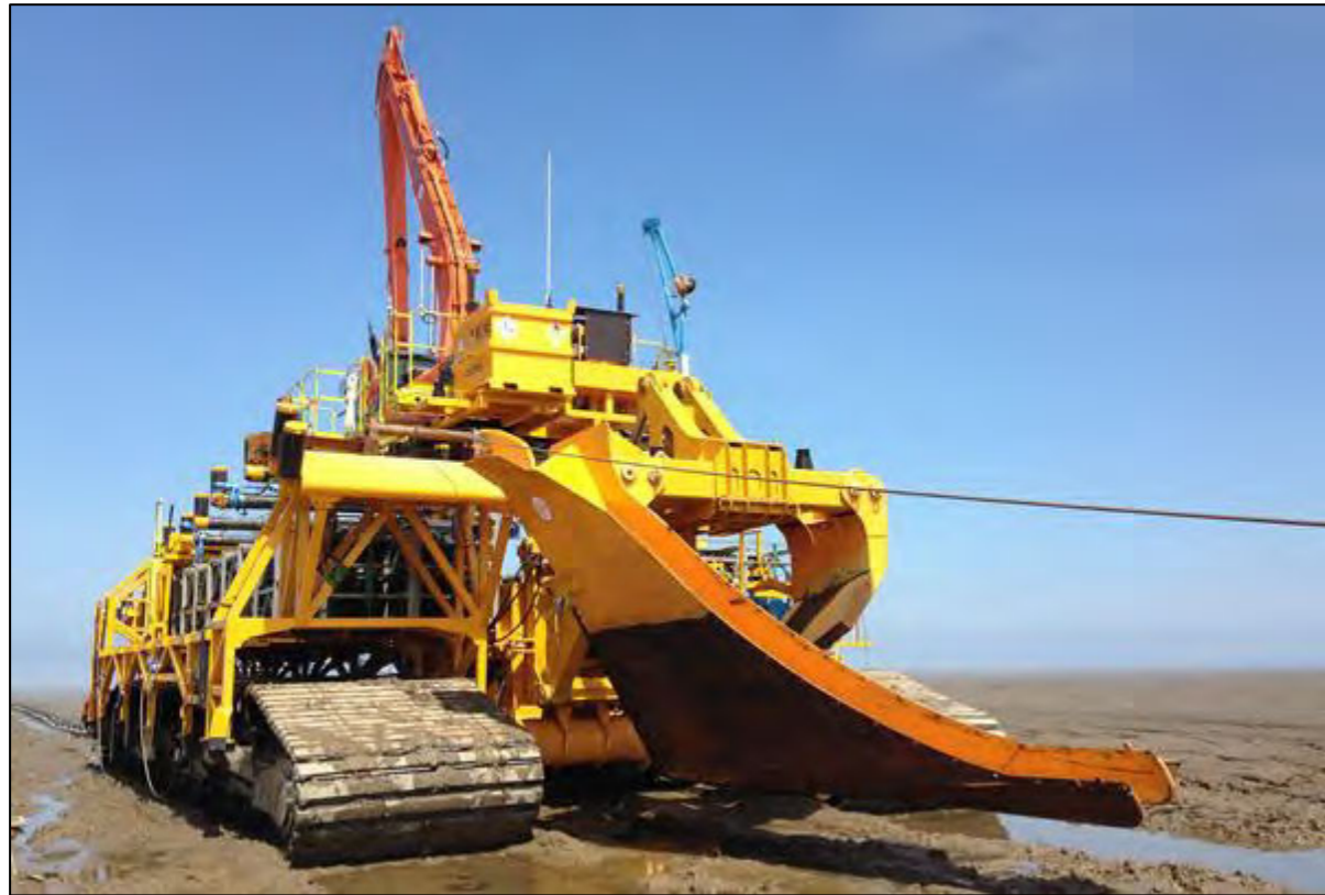
Figure 3.25: The 'sunfish' installation tool as used for cable installation at the Race Bank offshore wind farm.
