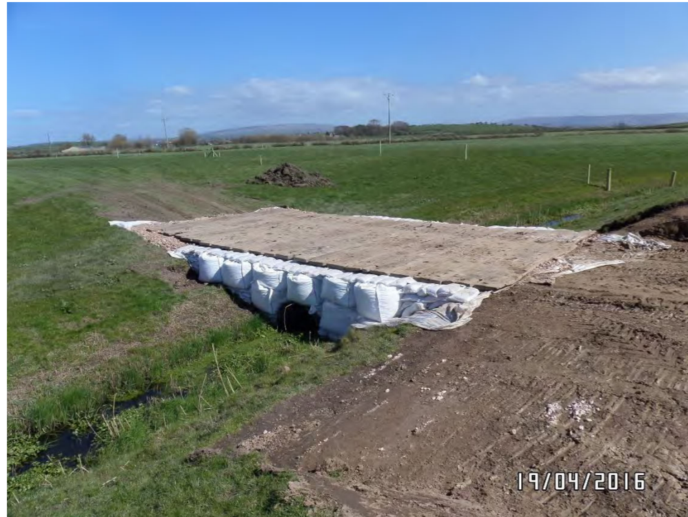
Figure 3.28: A sample flume installation.
